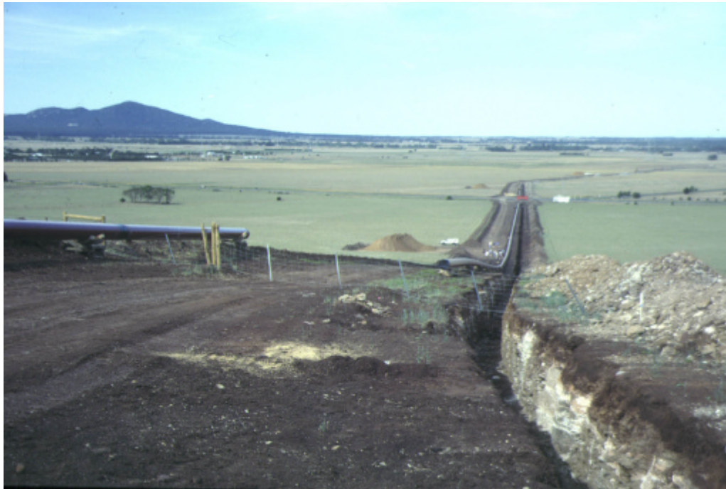
Lovely Banks monocline in the basalt plain, view eastwards (You Yangs on the left). The road running across the image is the Bacchus Marsh-Geelong road. SW101 is situated in the pipeline trench near the road crossing
